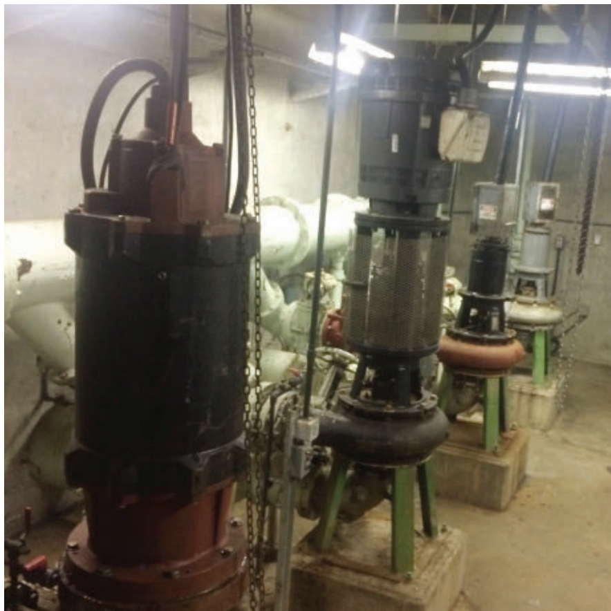
The Sewer Authority Mid-Coastside (Half Moon Bay, Calif.) installed an anti-ragging device in one of its pump stations. Sewer Authority Mid-Coastside (Calif.)
