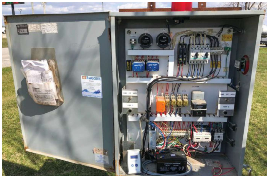
Image 1. The installed pump monitoring system is designed to prevent ragging with early detection. (Image courtesy of Deragger Inc.)
